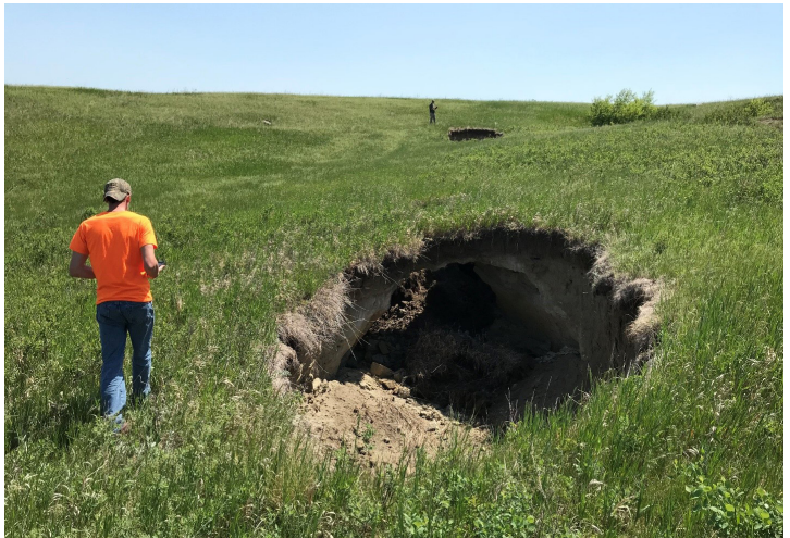
Sinkhole on Game & Fish property near Beulah. Visible sinkholes are part of the same room that is collapsing.
